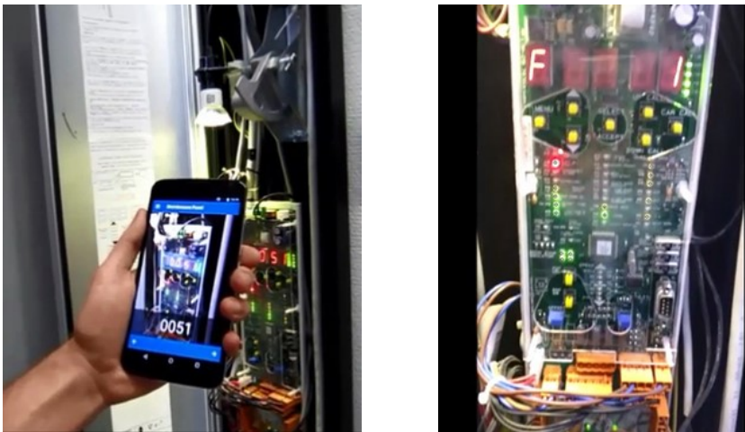
Fig. 4. The demonstrator: On the left, mobile application, (Fault 51 detected). On the right, image of detected maintenance panel with LEDs recognized.
